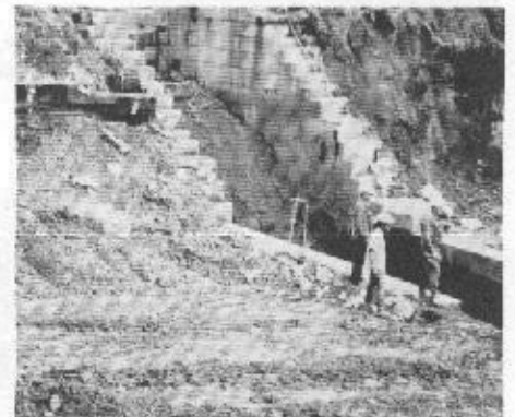
Dismantling of Locks #2 and #3. Note the height of the lock, dwarfing the workmen below.
