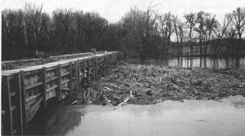
Debris piled against the Monocacy Aqueduct
