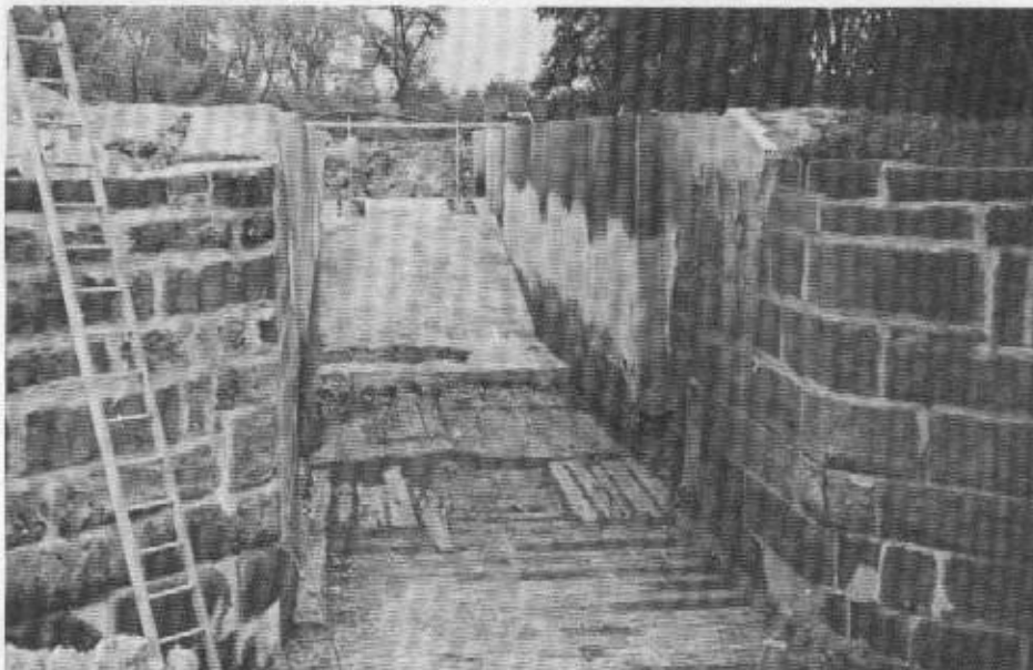
Recent photo of O. & E. Canal Lock No. 40, near Republic Steel's Cleveland plant. (Courtesy Bruce Anderson and Gary Course.)
