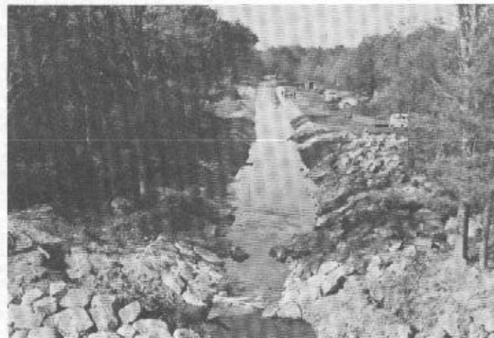
View of the restored section of canal from the new bridge. Much work still to be done.
