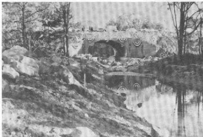
New canal bridge, built by Massachusetts Dept. of Public Works for route #129. Towpath will be at left.
