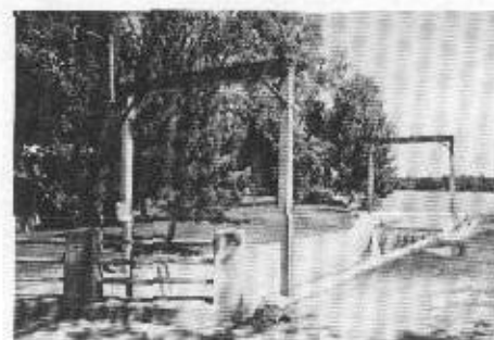
Close-up of one of the two WPA locks built in 1937 to connect Muskrat Lake (in the background) with Lake Sallie at the site of the old Dunton Locks built 1888. Bev Morant thinks the steel structures were built to house guillotine gates.
