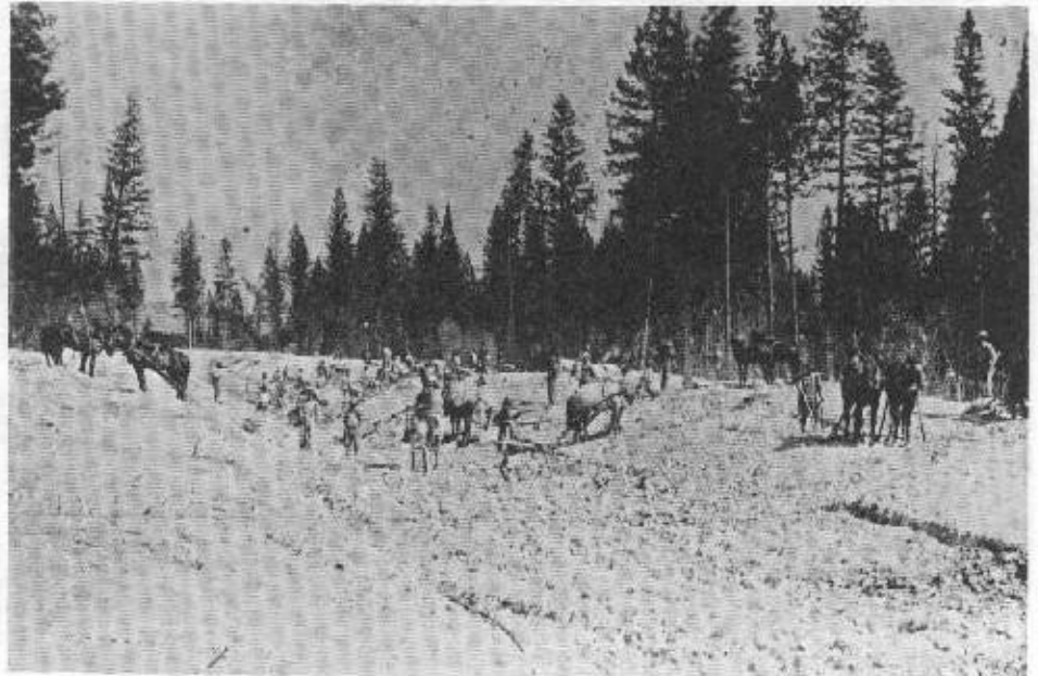
Construction of the Baillie-Grohman Canal at Canal Flats, British Columbia underway c1888. (Mrs. Mabel Jordon and Vice-Admiral Baillie-Grohman)
