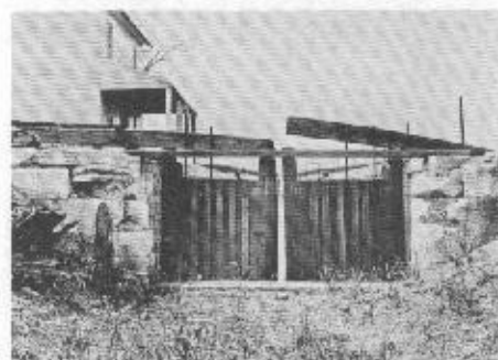
West end of the lock at the Mad River Aqueduct in Dayton, March 23, 1911. The canal channel had been dry for a few years when this photo was made; wood-work of gates still in good shape.
