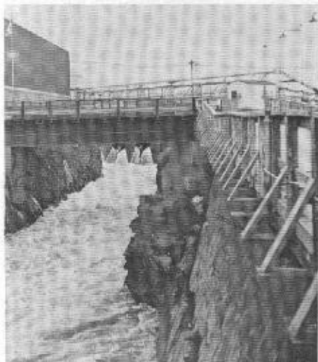
Rock excavation for the unfinished lock at Fort Francis, Ontario. Now used as waste water channel for a paper mill. For a century this lock has been discussed, and investigated, but never completed. (Photo by Robert Legget.)
