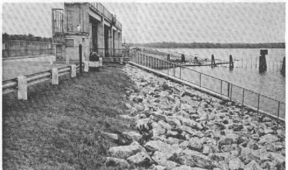
End view of Rodman Dam on the Cross-Florida Barge Canal, with Lake Oklawaha to the right. (Gould photo).
