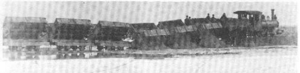
Building bank across slough on ice showing narrow gauge train with six cars dumped. January 23, 1903. (Photo courtesy of the Rock Island District, Corps of Engineers.)
