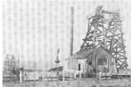
Excavation at Mile 22, Eastern section of the Hennepin Canal, showing the cableway, towers and bucket specially constructed for this problem area of canal prism. December 10, 1904. (Photo courtesy of the Rock Island District, Corps of Engineers.)
