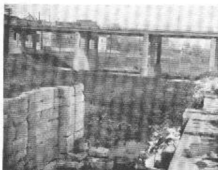
The downstream end of Lock 14 on the Illinois-Michigan Canal being restored by volunteers. (Photo by R. F. Whalen.)
