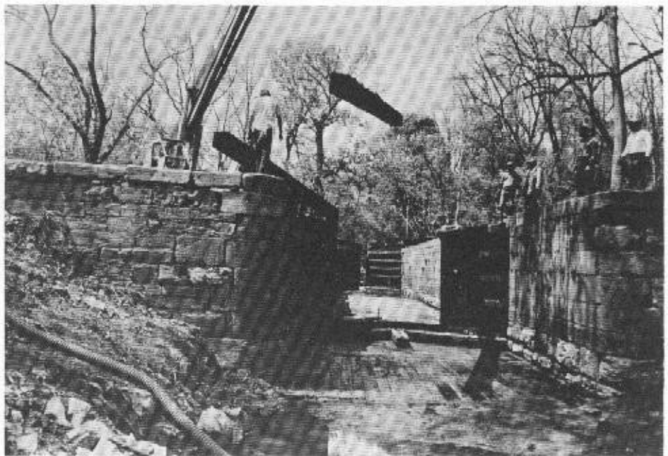
New, mitre-type wooden gates and balance-beams are shown here being installed at Lock Number 47 of the restored Union Canal section west of Reading. This is a project of the Berks County Parks and Recreation Board.
