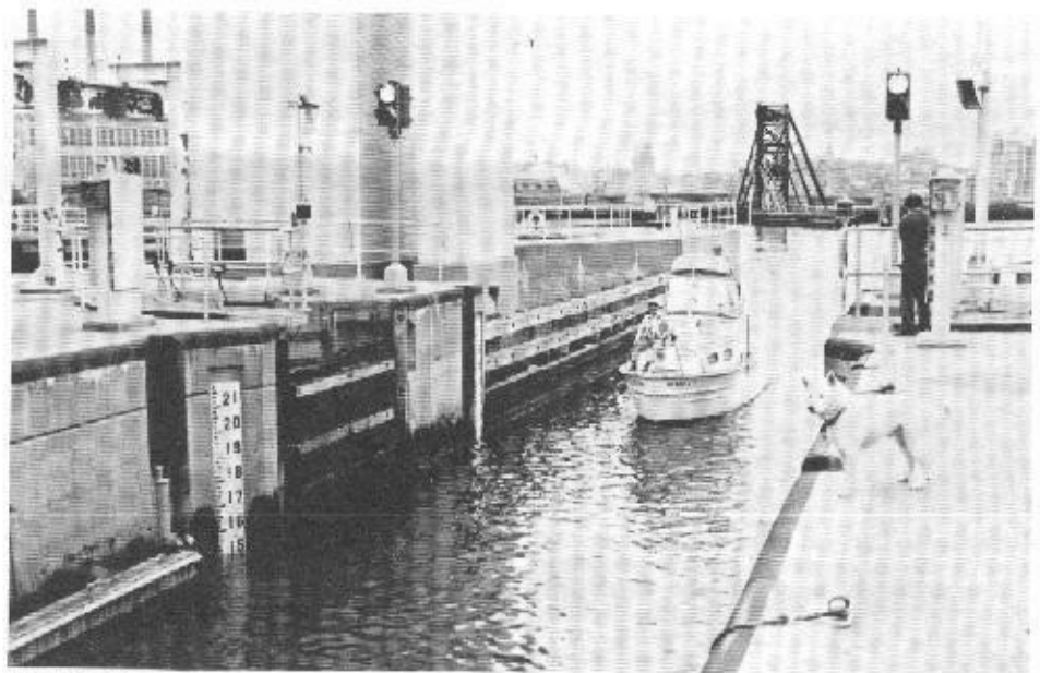
The Amelia Earhart Locks at Dam Site are located on the Mystic and Malden Rivers in both Everett and Somerville, Massachusetts. There are three locks at this site, all completed in 1966. This view shows Lock #2, one of the two small locks, which is 120' long and 25' wide. The commercial lock (not shown) is to the left and is 325' long and 45' wide. (Alden Gould, Director, ACS)
