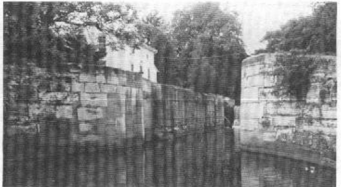
A well preserved lock on the old Illinois and Michigan Canal at Channahon State Park, near Chicago.
