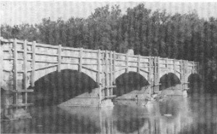
Monocacy Creek Aqueduct on the Chesapeake and Ohio Canal close to the Montgomery County and Frederick County Line in Maryland. Note stabilization work on the old masonry.
