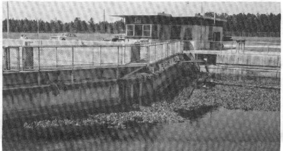
Inglis Lock on the Cross-Florida Barge Canal, 84 x 600 feet, built in 1970. This view shows the east gate and control building. Note the "Hyacinths" floating in the lock chamber. (Photo by Alden Gould, March 1975)
