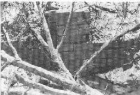
Remains of Guard Lock on Kankakee Feeder, most of which was timber construction.
