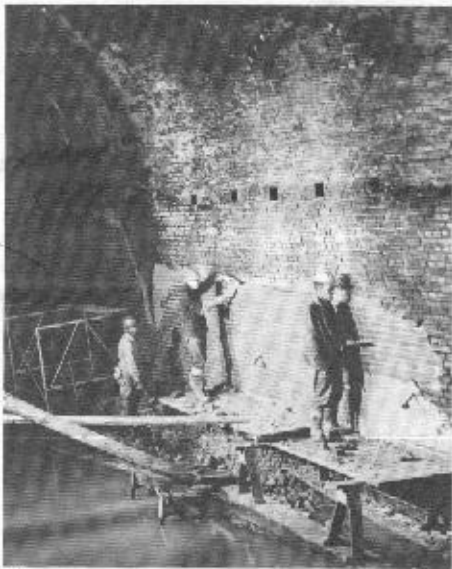
Masons at work on the interior of the tunnel as part of a National Park Service project in the 1960's. (National Parks Service Photo)
