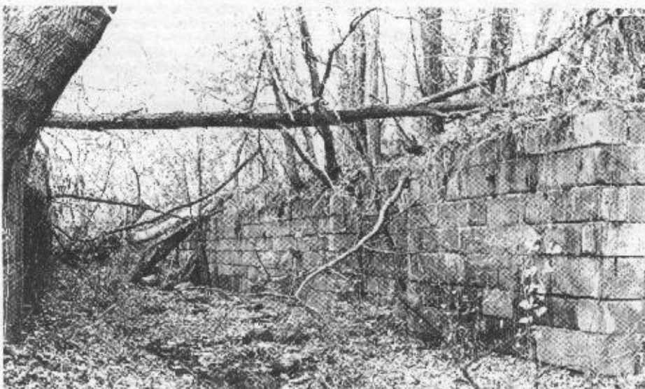
Virtually in the shadow of the Three-Mile Island cooling towers, this well-preserved lock on the old "Main-Line Canal" is located about a mile south of Middletown, Pa. Its somewhat isolated location has preserved it from vandalism and the inroads of a nearby branch of the Penn-Central RR., which has almost destroyed "Buck Lock" a mile or so further south. Falmouth Lock, a deep lock at the lower tip of Three-Mile Island is in almost as good shape as the Middletown Lock. (Photo by Bill Shank, 1980)
