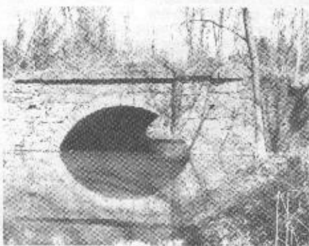
Opossum Creek Culvert below Lynchburg, completed in 1840, second largest of the culverts between Richmond and Lynchburg. (Courtesy of John Taylor.)
