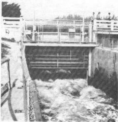
Upper vertical gate of the West Palm Beach Canal lock (135' x 25') just above tidewater. The lock is not operational. It was a part of one of the main canals serving for drainage and navigation in the early 1900's (Photo by Alden Gould)
