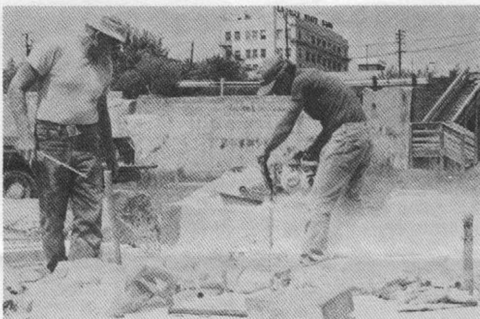
Stone-cutters continue the restoration process for Lock 14 near the terminus of I & M Canal in LaSalle. This $226,000 project, funded by the Illinois Department of Conservation and a National Park Service Maritime Grant, will restore the lock to historically accurate working order. Site restoration and interpretive signage are being planned. (Courtesy Upper Illinois Valley Assn., photo by LaSalle Daily News-Tribune).
