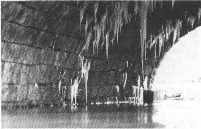
FIGURE 6—BURNETT'S CREEK ARCH, 1974: VIEW LOOKING NORTH FROM WATER LEVEL INSIDE THE ARCH, SHOWING ICICLES AND COURSES OF STONE
