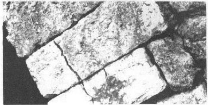
FIGURE 2—CRACKED RING STONES, BURNETT'S CREEK ARCH, 1974: COMPRESSION FRACTURES ARE VISIBLE IN RING STONES ON WEST PART OF THE NORTH PORTAL Courtesy of Author.
