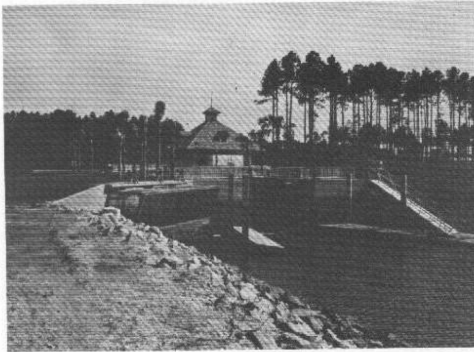
Two-way lock at Waxford Plantation, Hilton Head, South Carolina. Looking into the lock from the outer entrance.
