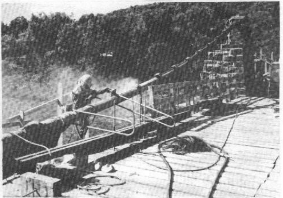
Blasting the accumulated dirt, rust and paint off the old cable wires before re-wrapping them. The "trombone" coils near the operator are the old floor support devices which had to be removed, and replaced as the cable cleaning and re-wrapping progressed.
