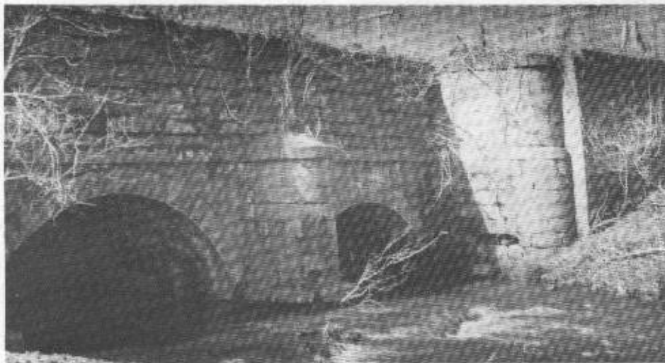
Allegheny Creek Aqueduct, south of Reading. The Schuylkill Greenway Association is cooperating with the Berks County Parks Authority to stabilize the old aqueduct and make it part of a canal park. (Bruce Russell photo.)
