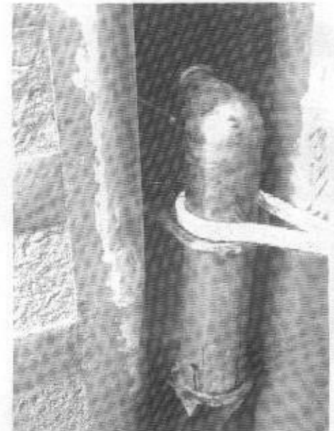
The floating "bollards", to which the boats are hitched in the lock, rise and fall with the lock water level, eliminating the need for manual guide ropes to hold the boats in place against the lock walls.
