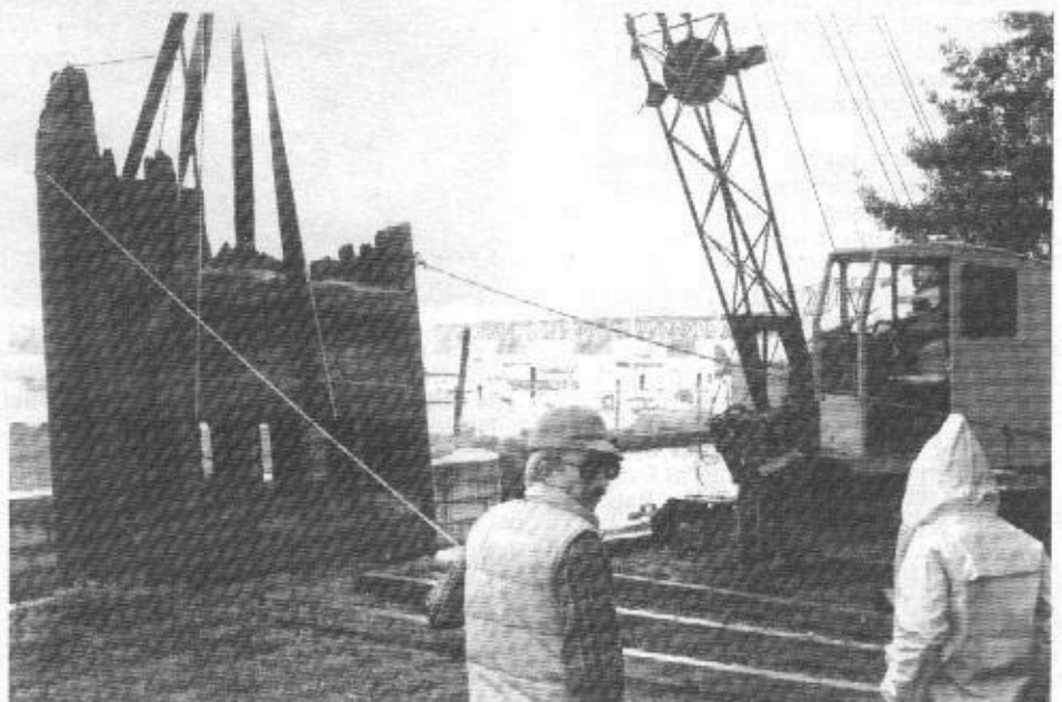
The old lockgate just after the "lift" out of the silt in the bed of the lock. In the foreground is C. Jay O'Dell, Project Coordinator, Maryland Tidewater Administration.
