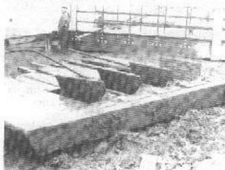
Lower end of the lock gate, placed on skids for examination and measuring. The old, metal "wicket gates" were all in the "open" position. One of the wicket-gate control rods (and handle) was fully intact, though slightly bent.
