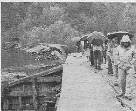
The badly-breached Three-Mile Dam, near Hunt's Lock on the Lehigh, is inspected in the rain by our hardy PCS members.
