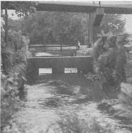
The control weir on the Canal Feeder adjacent to the new Dam at Allentown.
