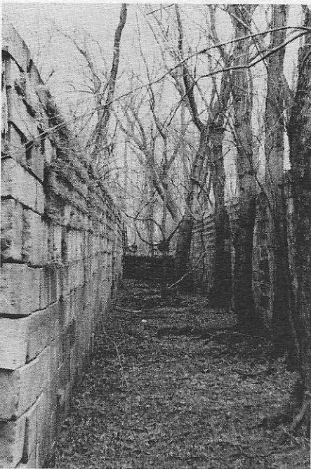
One of the best preserved locks on the Susquehanna Division is the Mahantongo Lock. The canal crossed the creek of the same name on an Aqueduct, just above this lock, whose piers are still standing.
