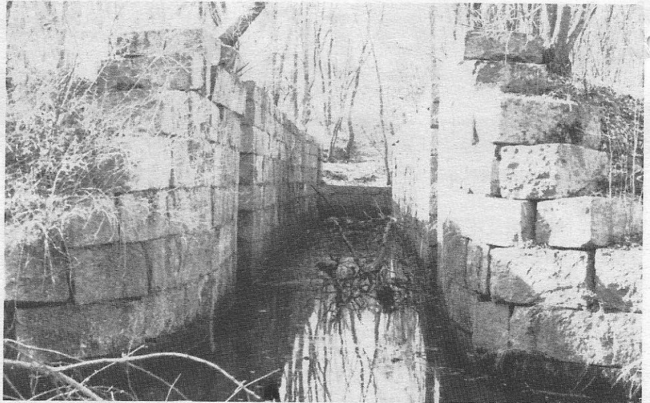
Blackstone Canal Lock below Millville, Massachusetts, looking into the chamber from the downstream end. (Photo by Dave Barber, 3/12/88.)
