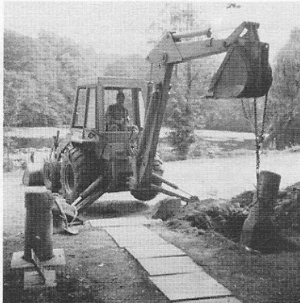
Delaware and Hudson Canal Snubbing Post being installed at Waterloo Village, New Jersey, close to the French Snubbing Post, previously acquired by Bill McKelvey. (McKelvey photo.)
