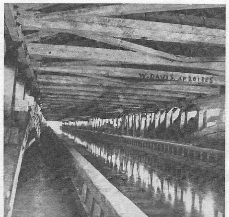
Interior of the Juniata Aqueduct, on the old "Main Line" near Amith Hall, about 1895.
