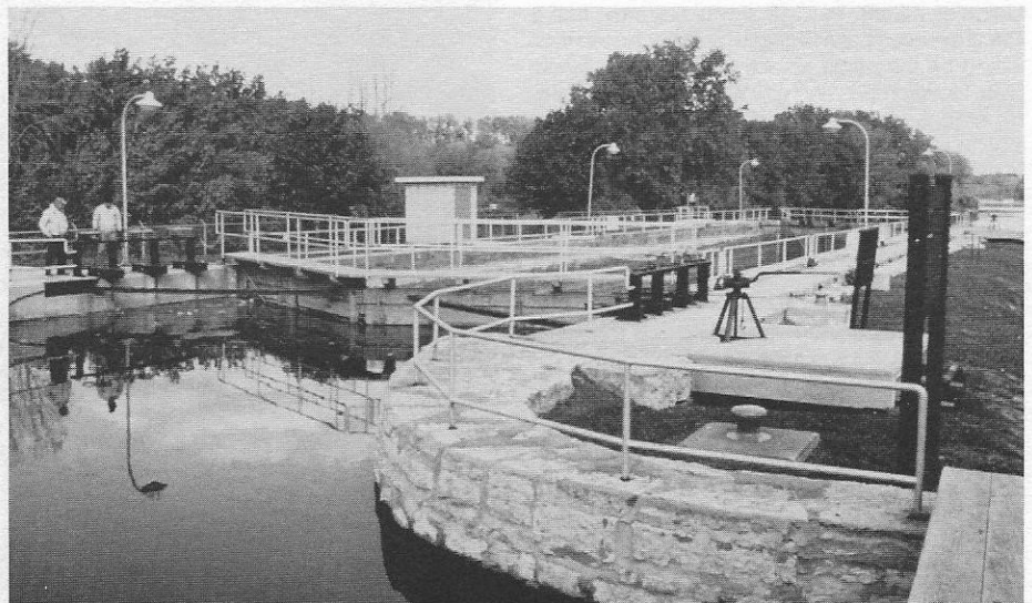
A Fox River lock, showing the turnstile for hand operation of the gates. Photographs courtesy of Kenneth J. Theine, Executive Director, East Central Wisconsin Regional Planning Commission.
