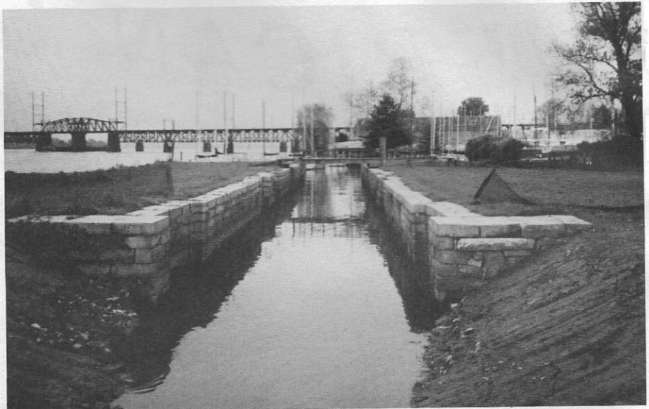
View from the top of the control weir, looking south into the tidelock of the S. & T. Canal, now cleaned out to almost its historic depth. Missing blocks from the sidewalls have been replaced and the walls reinforced.
