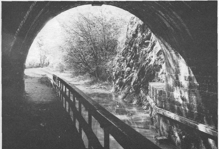
View of the west portal from inside the tunnel. Note the original wooden guardrail in the foreground, and the "rubbing rail" at the lower right, to prevent boats from coming in direct contact with the masonry tunnel wall.
