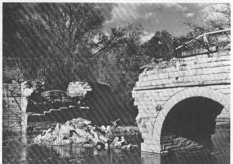
1972 Hurricane Agnes, collapsed after two days of heavy rains. About 70 feet of the aqueduct, including the central and small upstream arches (there were three arches), were washed into the stream. This is the second aqueduct to have collapsed in the past two years. Seneca Creek Aqueduct (mile 23) collapsed in September 1971.
