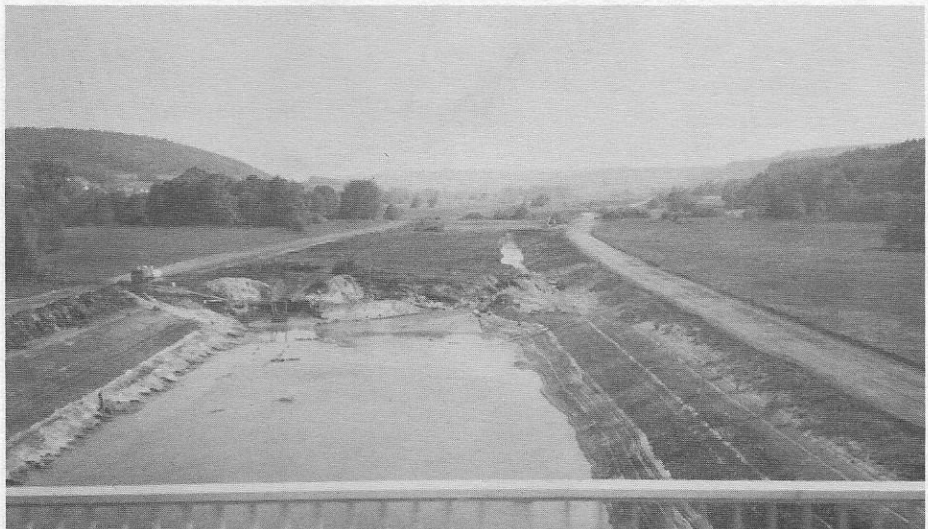
Construction on one of the final, level sections of the Main-Danube Canal, below the Berching Lock. (Photo by Roger Squires, May of 1990.)
