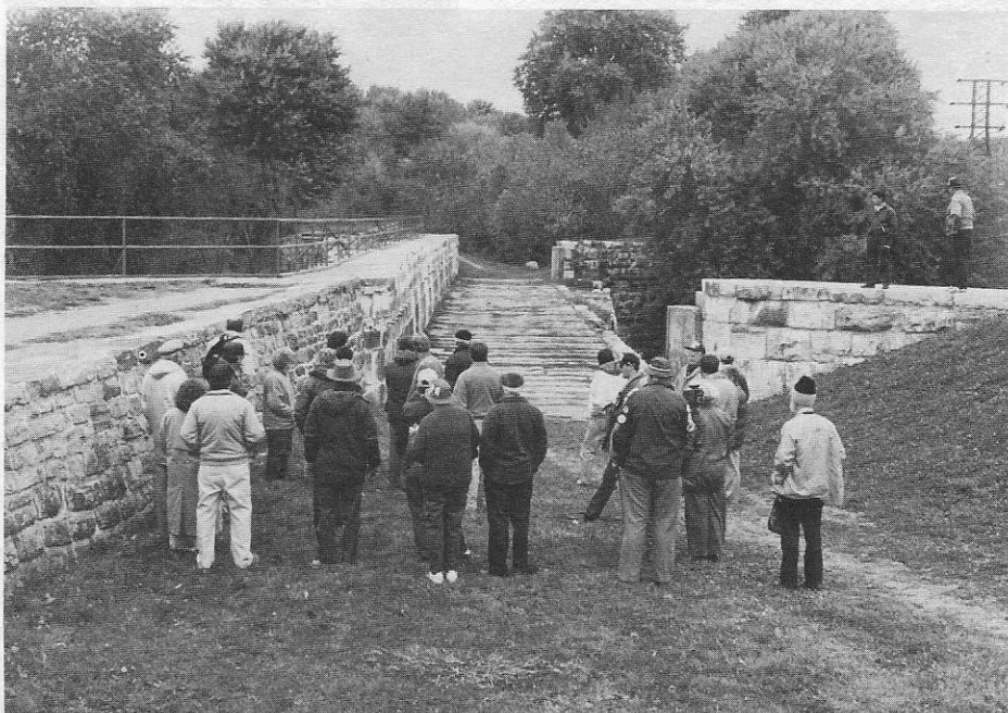
The C and O Canal Aqueduct across the Conococheague Creek at Williamsport, Maryland. The upstream wall collapsed shortly before the canal was abandoned, and it was never rebuilt.
