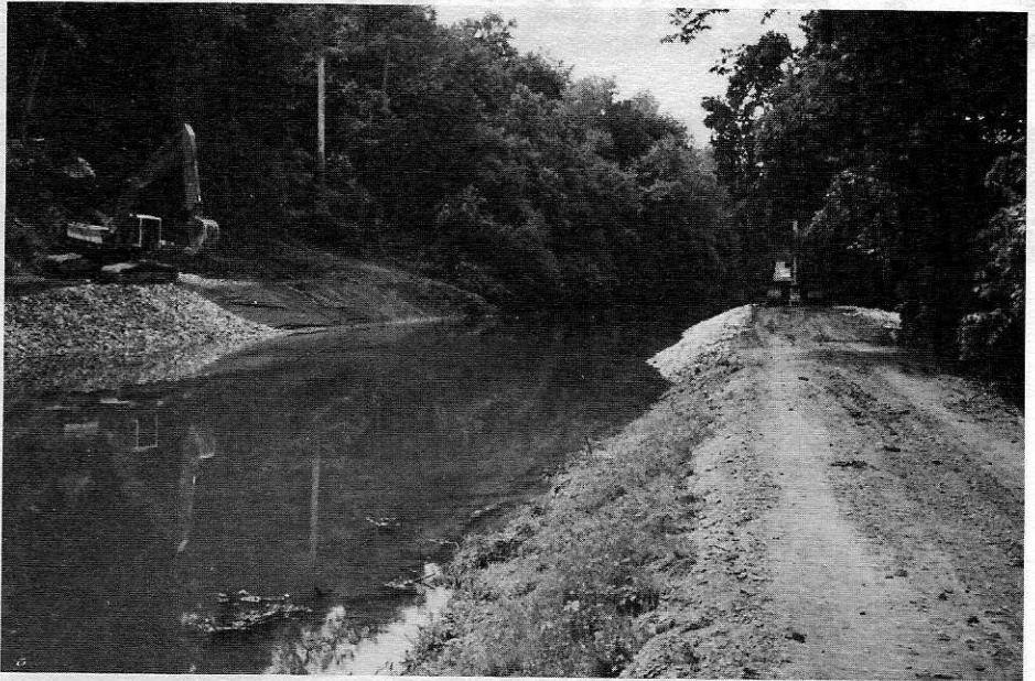
Utility crews work on canal banks to stabilize the repairs made at the site of the towpath break. (June 1992)
