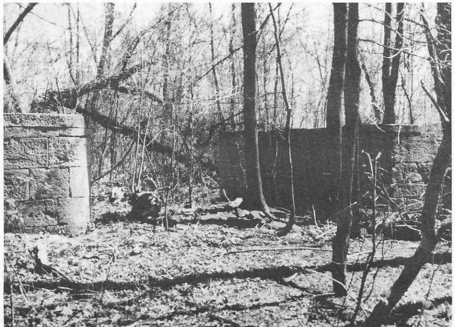
Scottsville Feeder Gates —Allen's Creek (Now Oatka Creek) waters were impounded by an arched dam just to the right and sent down the Scottsville Feeder through these gates. This was one of four sites where the Genesee River was tapped for water for the canal. Iron gatepost collars are still in place.
