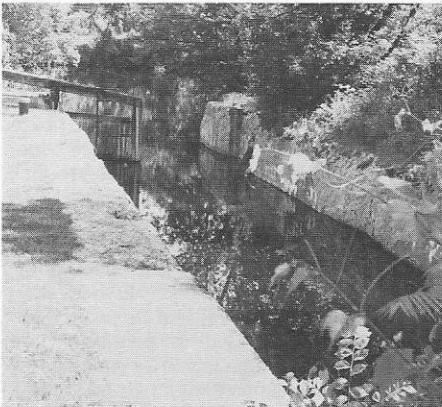
At Schuylerville, we discovered one of the locks of the old Erie Canal in fair state of preservation. One of the old wooden, hand-operated lock gates was still in place.
