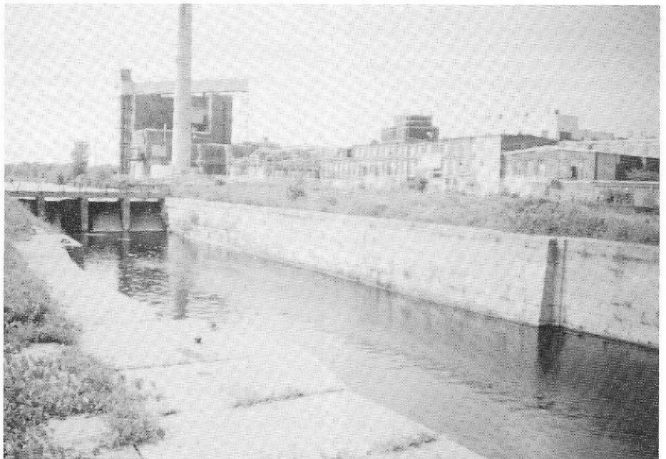
Cornwall Canal, North chamber of second lock below power dam, looking west.
