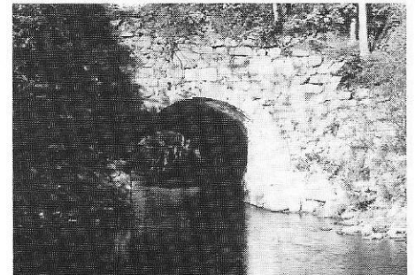
We visit a well-preserved culvert under the Morris Canal near the west end of the waterway.
