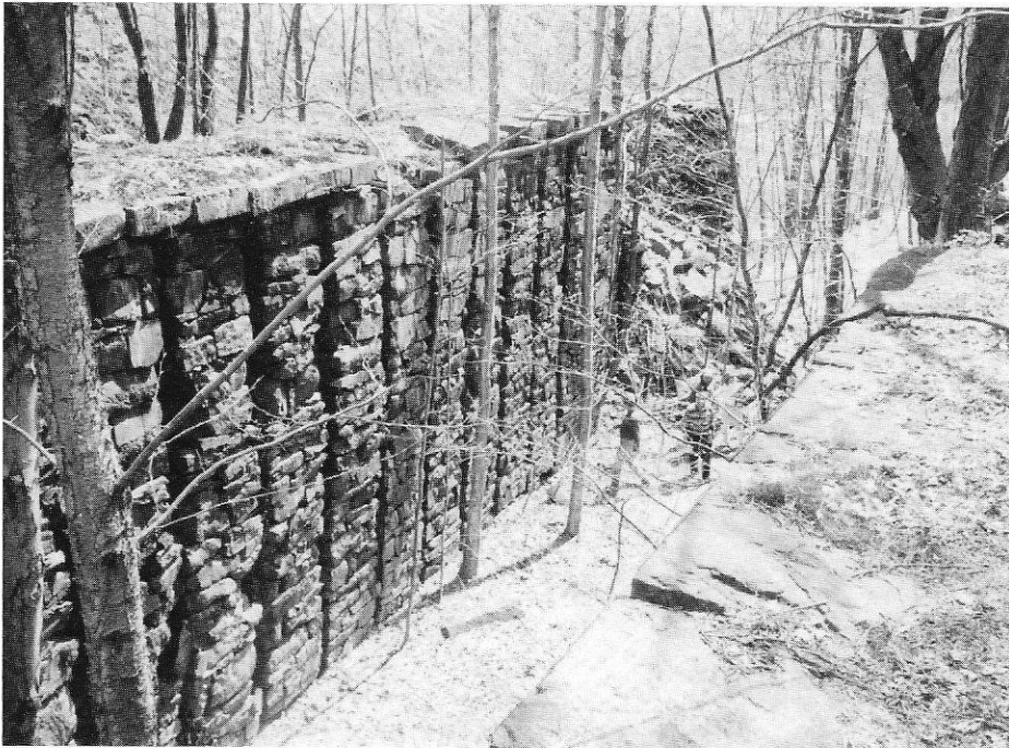
Ruins of the tremendous Lock Number 28 on the Upper Lehigh Canal, with a lift of thirty feet. Two floods forced the abandonment of the Upper Lehigh Canal. (Denver Walton photo.)
