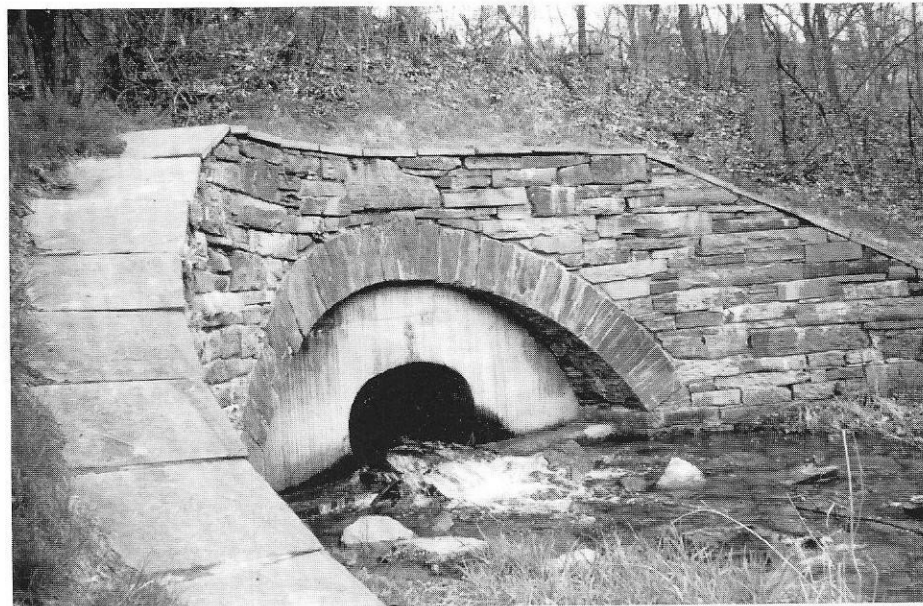
Well-maintained culvert under the Chenango Canal at Chenango Valley State Park, Chenango Forks, N.Y. (Linda House photo)
