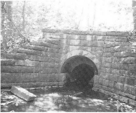
One of the 1850 stone culverts of the embankment of the Enlarged Erie Canal near Holley, NY. A well-built structure made of cut limestone blocks.
