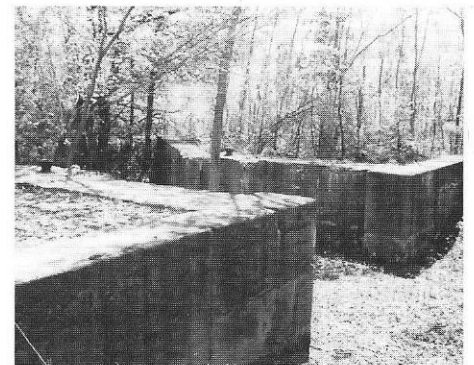
Entrance to the Junction Lock at Greece, NY. It was created as a temporary structure only, in concrete.
