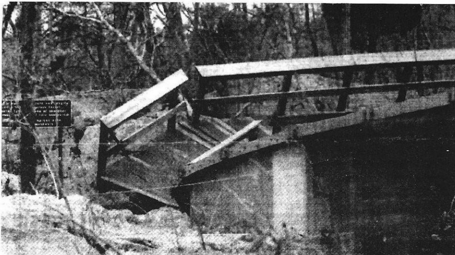
Typical recent flood damage to the C. & O. Canal. (Washington Post photo)
