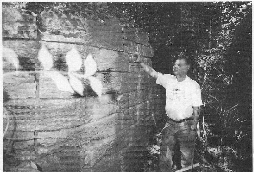
ACS president Terry Woods inspects the dressed stone portion of the Cincinnati and Whitewater Composite Lock Two
