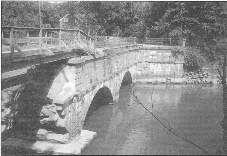
The Seneca Creek Aqueduct suffered more severe flood damage.
