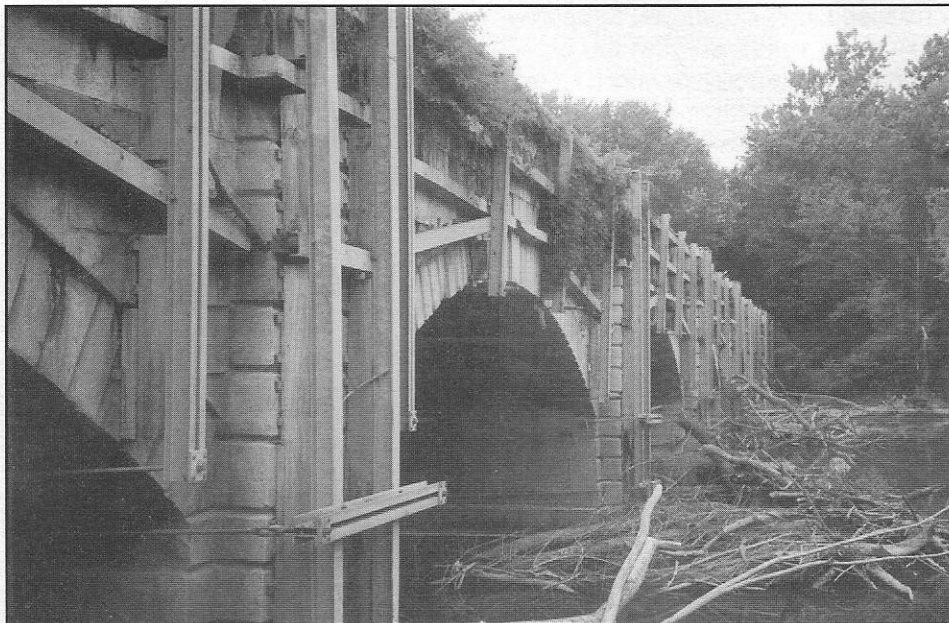
Temporary supports have held the aqueduct together since the assault of the 1972 hurricane.
