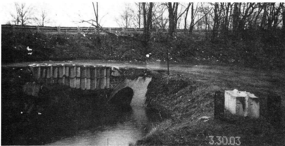
Culvert at Tyburn Road, looking north, on the Delaware Canal. Photo by David Barber.
