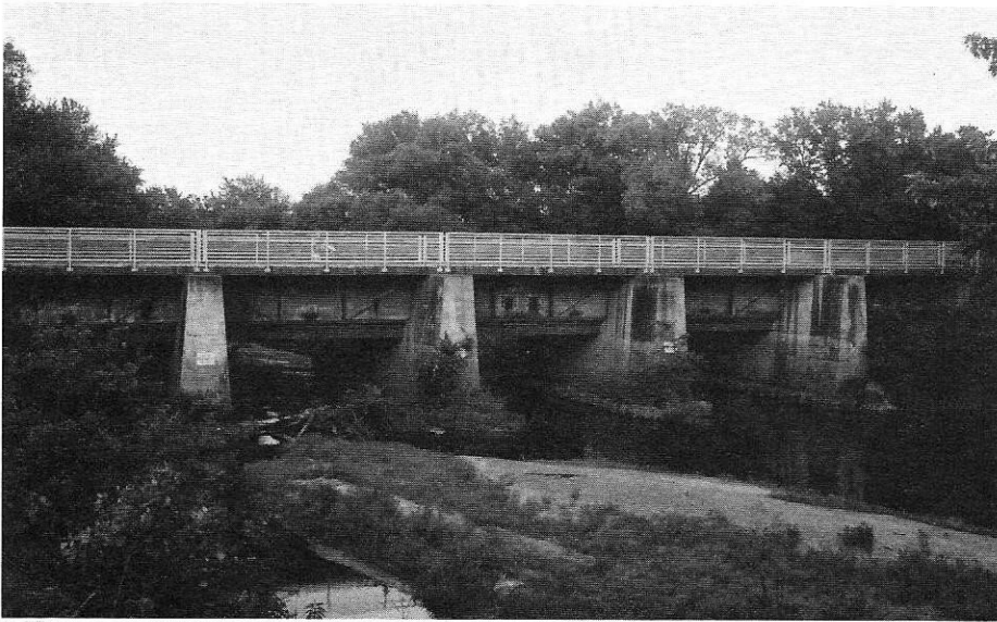
Aqueduct #9 carries the feeder canal over the Green River. Five of the original nine aqueducts are still in use. Photo by Mark Beech
