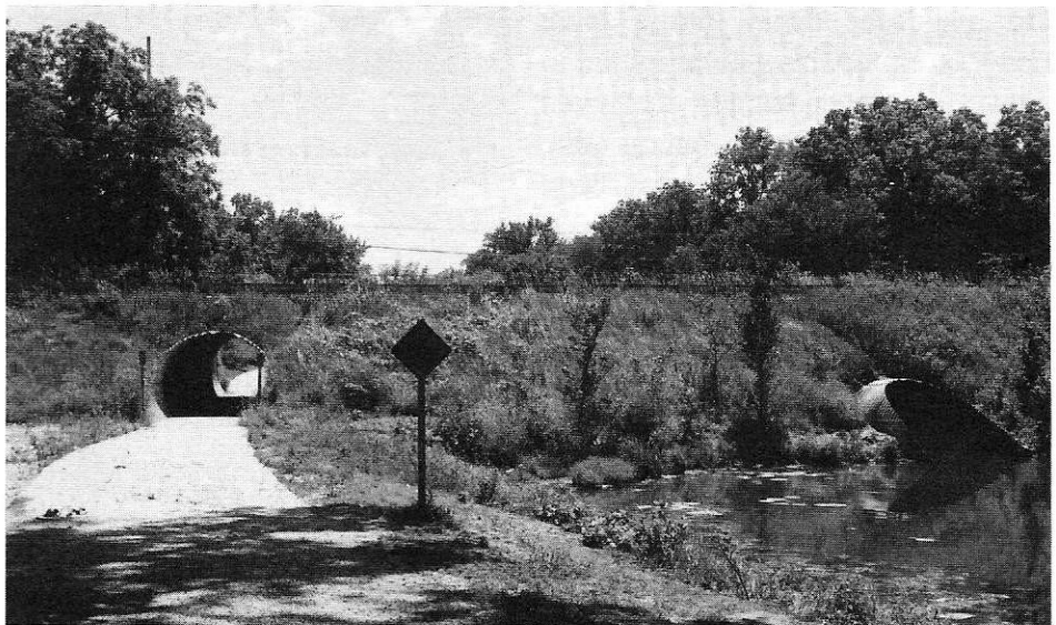
Just west of Lock #24, this road crossing shows the typical arrangement of one culvert for the trail and another (far right) for the canal. Photo by Mark Beech
