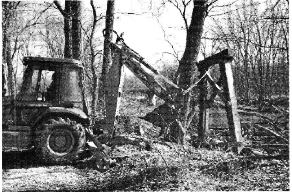
City Parks employee Dennis Morrow uses the backhoe to upright the A-Frame. Photo by Dan McCain.
