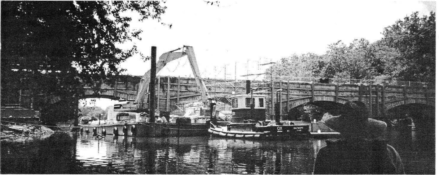
Upstream side of the Monocacy Aqueduct in the summer of 2003. The contractor is fully staged for restoration work. Note the array of equipment deployed for the task: barges, excavator, tugboat, etc.
