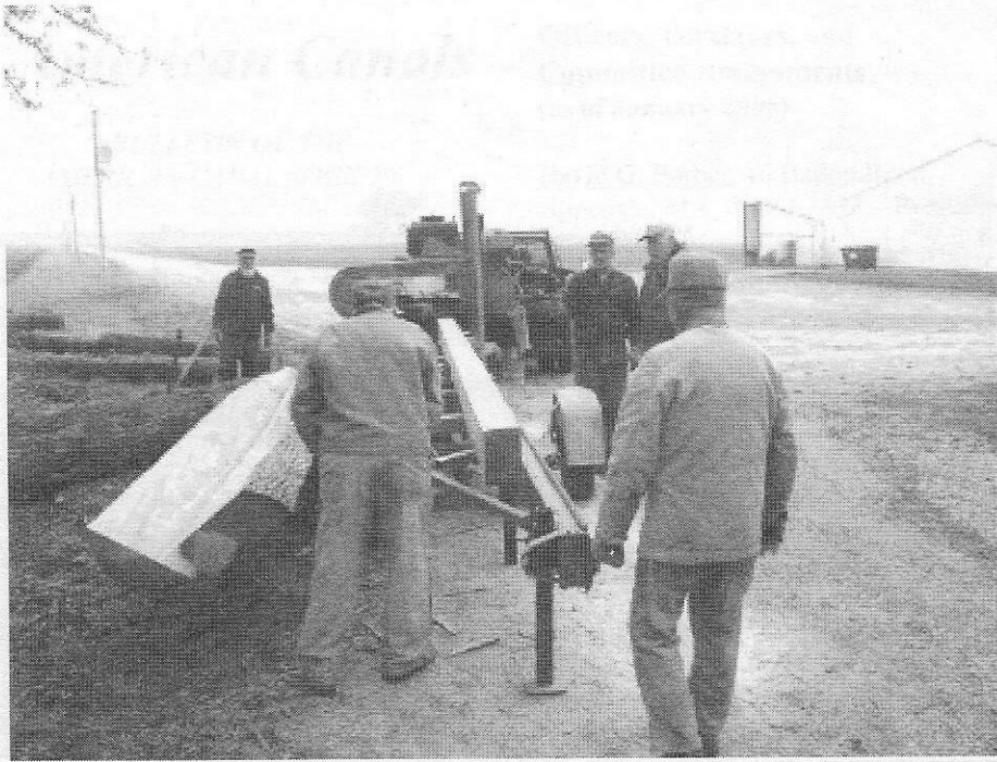
The volunteer crew cutting 6 x 8 and 8 x 8 inch timbers to be used as “blocking” to support disassembled bridge components.
