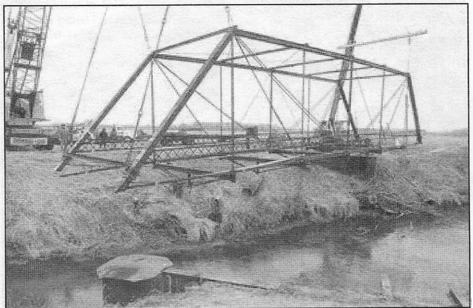
The Stearns Truss is removed by cranes from its place over Big Monon Ditch.
