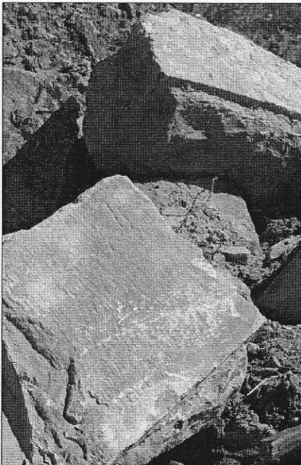
Hammer and chisel marks from the early 1800s can be seen on the stones that used to be part of Culvert 151 under the Wabash and Erie Canal. Jim Avelis, the Tribune-Star
