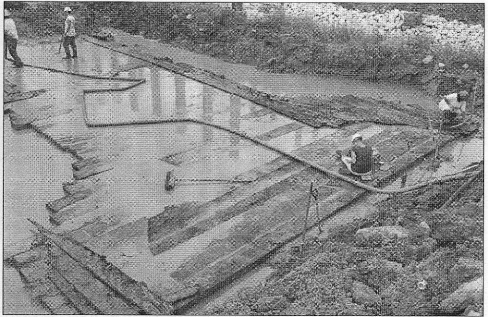
What lies beneath: Walsh Construction company workers clear mud and silt from the timbers of Culvert 151 in September. The 170-plus year old timbers will be removed and made part of a historical exhibit. Jim Avelis, the Tribune-Star
