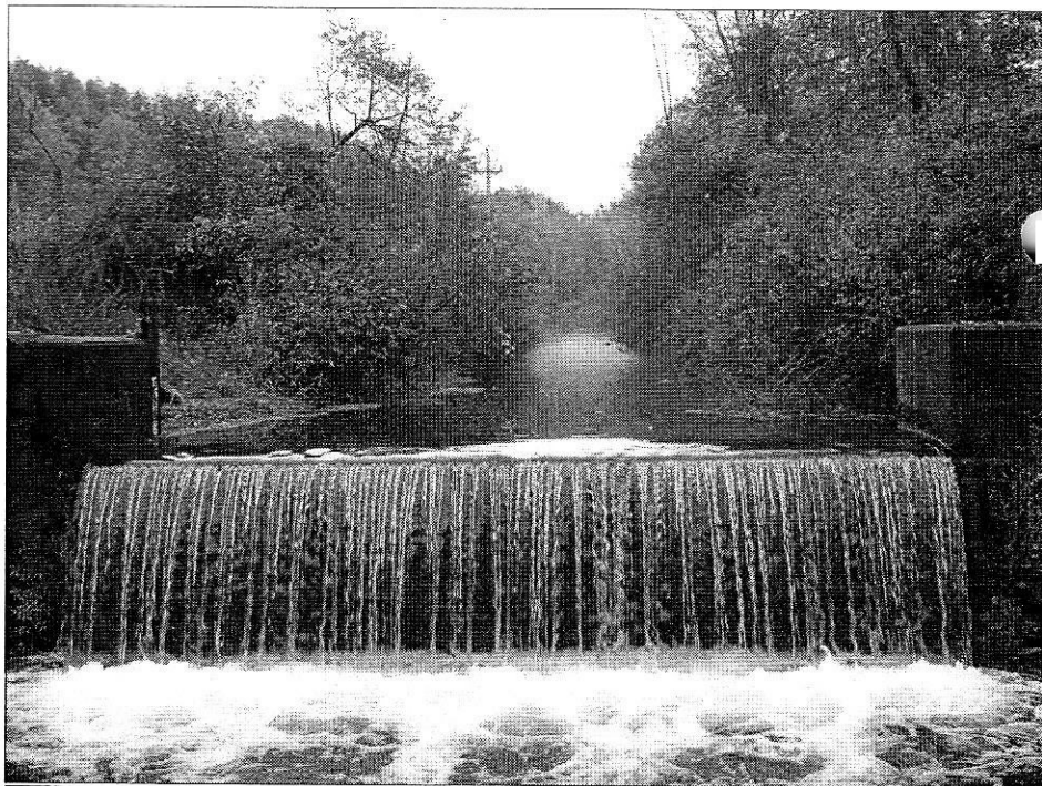
Abutment of Oriskany Aqueduct over the Oriskany Creek. Photo by Jakob Franke
